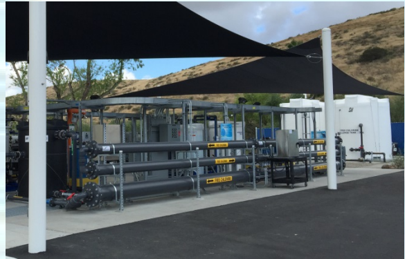
Padre Dam MWD Advanced Water Purification
